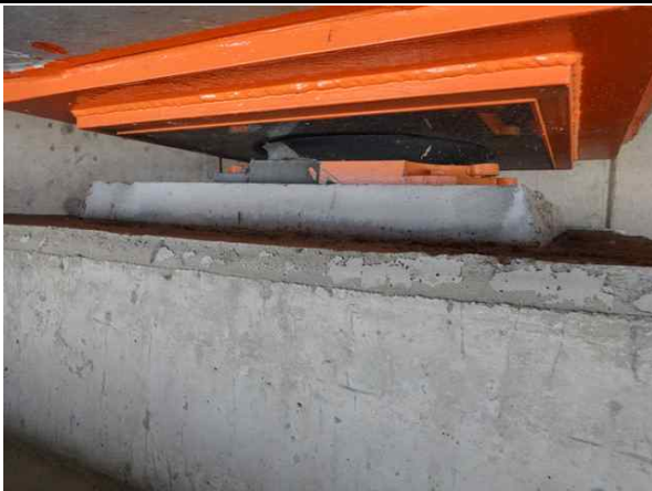
A1-Sh4 무수축물탈 균열(0.2mm/0.1m)
